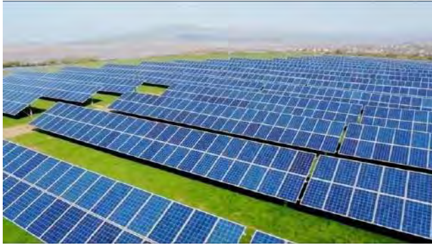
Gambar 3.7: PLTS Ground-Mounted (ESDM, 2019)
