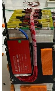
Gambar IV 10 Battery Management System (BMS) 24s 72V
