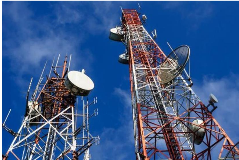
Gambar 2.10 Tower Based Transceiver Station
